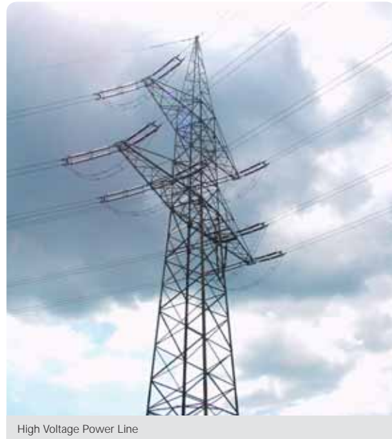
High Voltage Power Line
