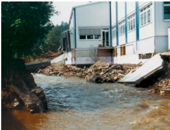
Fig. 19: Destroyed revetment of the Müglitz stream in Glashütte, 2002 (photo: LTV, 2002)
