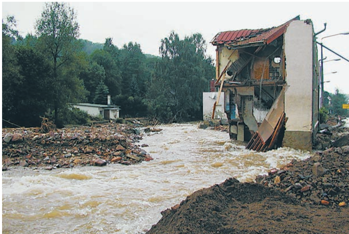
Fig. 8: Destroyed building and channel displacement of the Rote Weißeritz in Schmiedeberg (photo: GOTTFRIED HEROLD, 2002)
