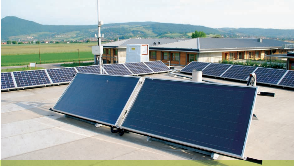
PV panels on the roof of the Energy Advice Centre
