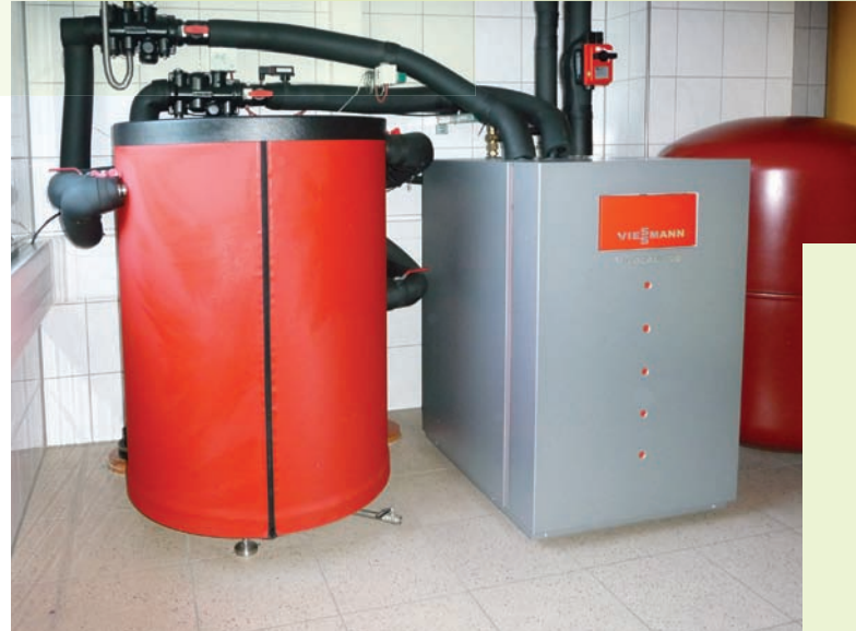
Heat pump and heat exchanger
