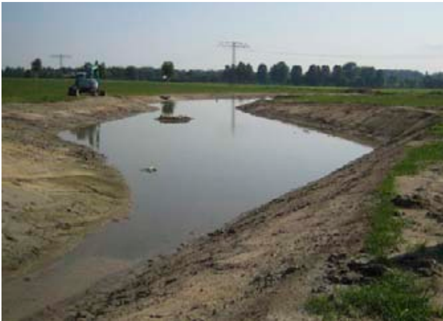
Water storage located in the construction; photo: S 177 OU Radeberg/GroBerkmannsdorf Community of Participants
