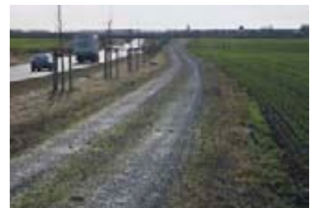
Creating a new access road parallel to the local by-pass; photo: S 177 OU Radeberg/GroBerkmannsdorf Community of Participants
