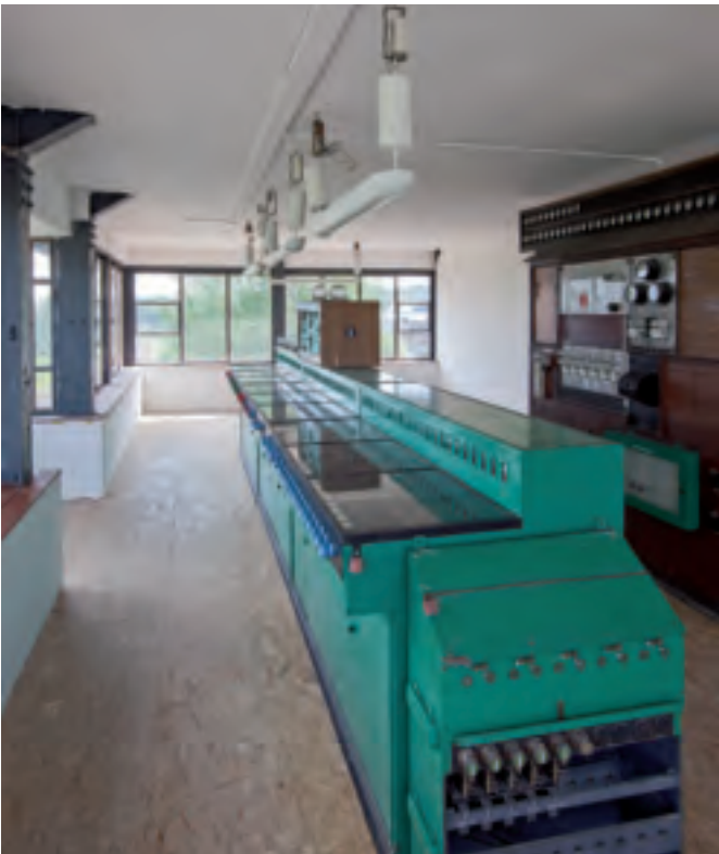
Switch tower 2 with electro-mechanical switching technology
