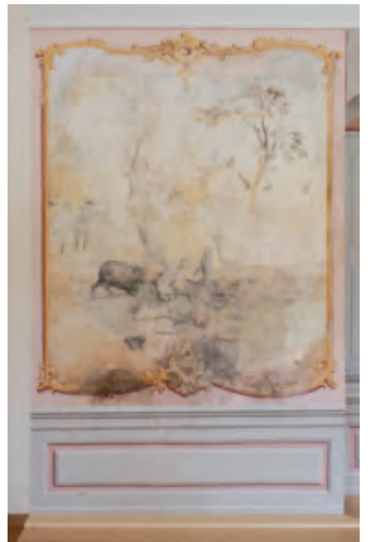
Mural on the upper floor after exposure
