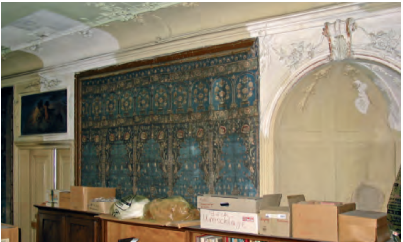
Section of the wall before the restoration with an alcove for an oven
